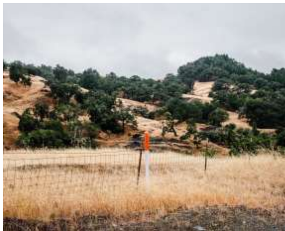
David Greer Underground fibre optic cable marker, Yorkville CA
