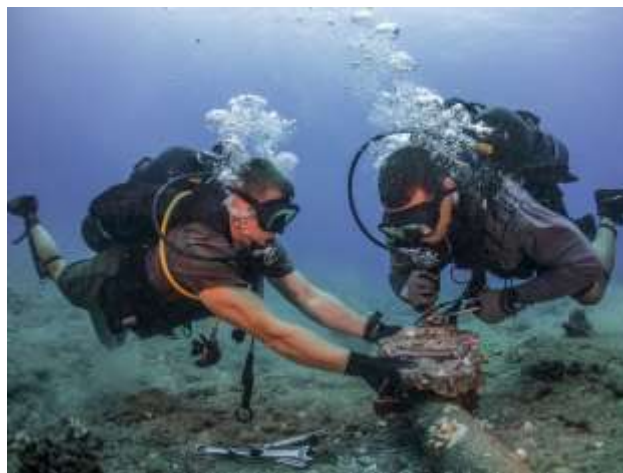
Flickr/Official U.S. Navy Page Divers remove corroded zinc anodes from an undersea cable near Hawaii.
