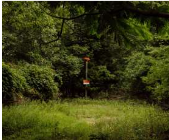
David Greer Underground fibre optic cable marker, New Jersey
