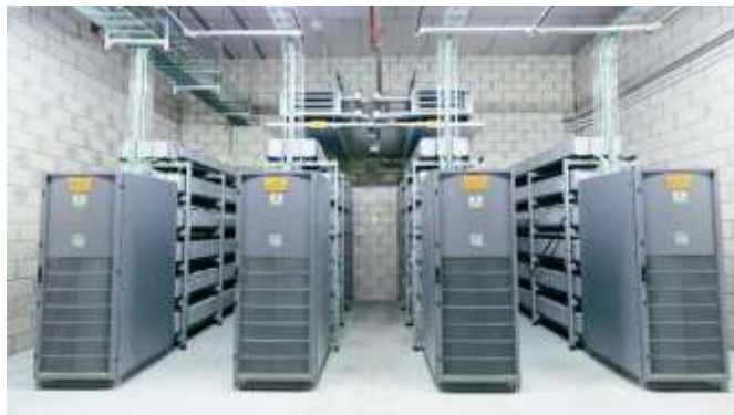
Timo Arnall/Vimeo Data center run by Telefonica in Alcalá, Spain
